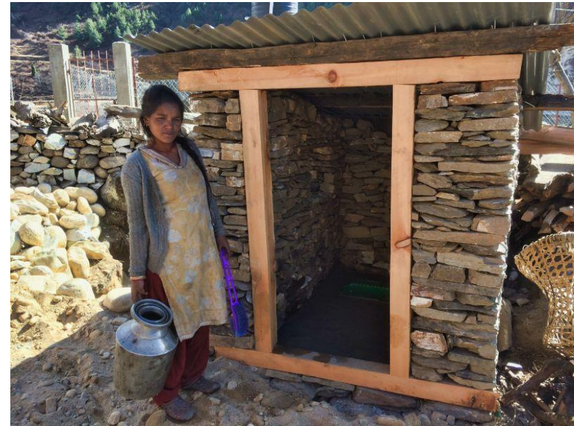
Pic.10. A Pit Latrine in Pere Village constructed as part of the GG1 project.
