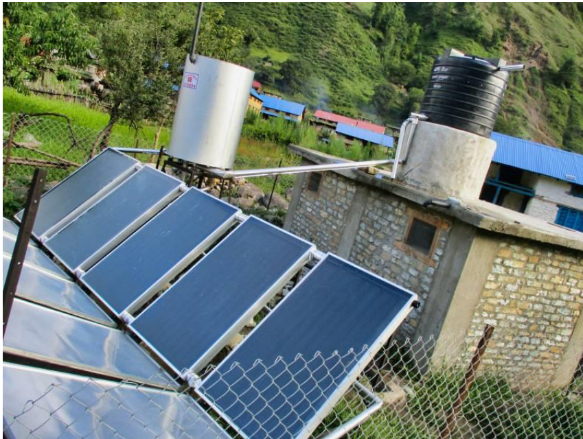
Pic.23. A view of SWHBC installed in Pere village as part of GG1.
