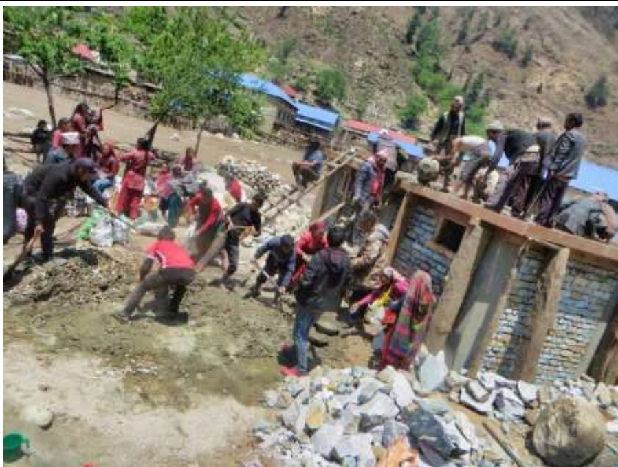
PIC.55. All Pere families help building their Solar Hot Water Bathing Center.
