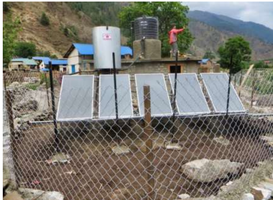
PIC.58. Solar Hot Water Bathing Center ready to use.
