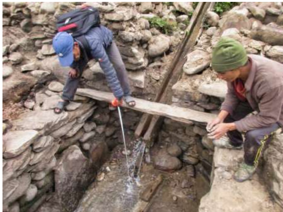
PIC.43. Land measuring and clearing for the new Improved Water Mill (IWM).
