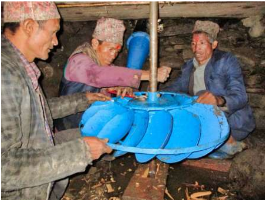
PIC.49. The new to install metal turbine of one of the IWM is mounted.
