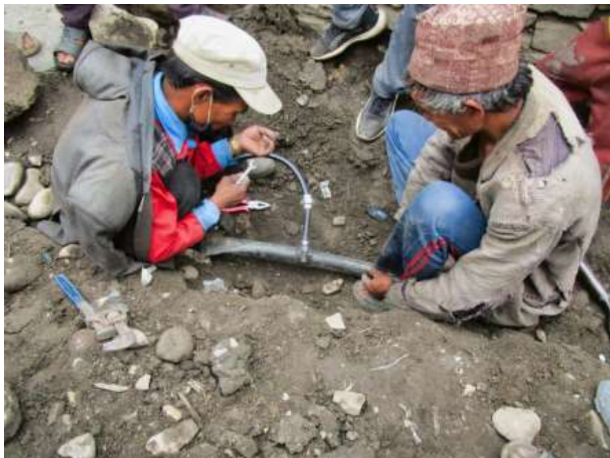
PIC.15. Pere people are learning how to repair and maintenance their DWS.
